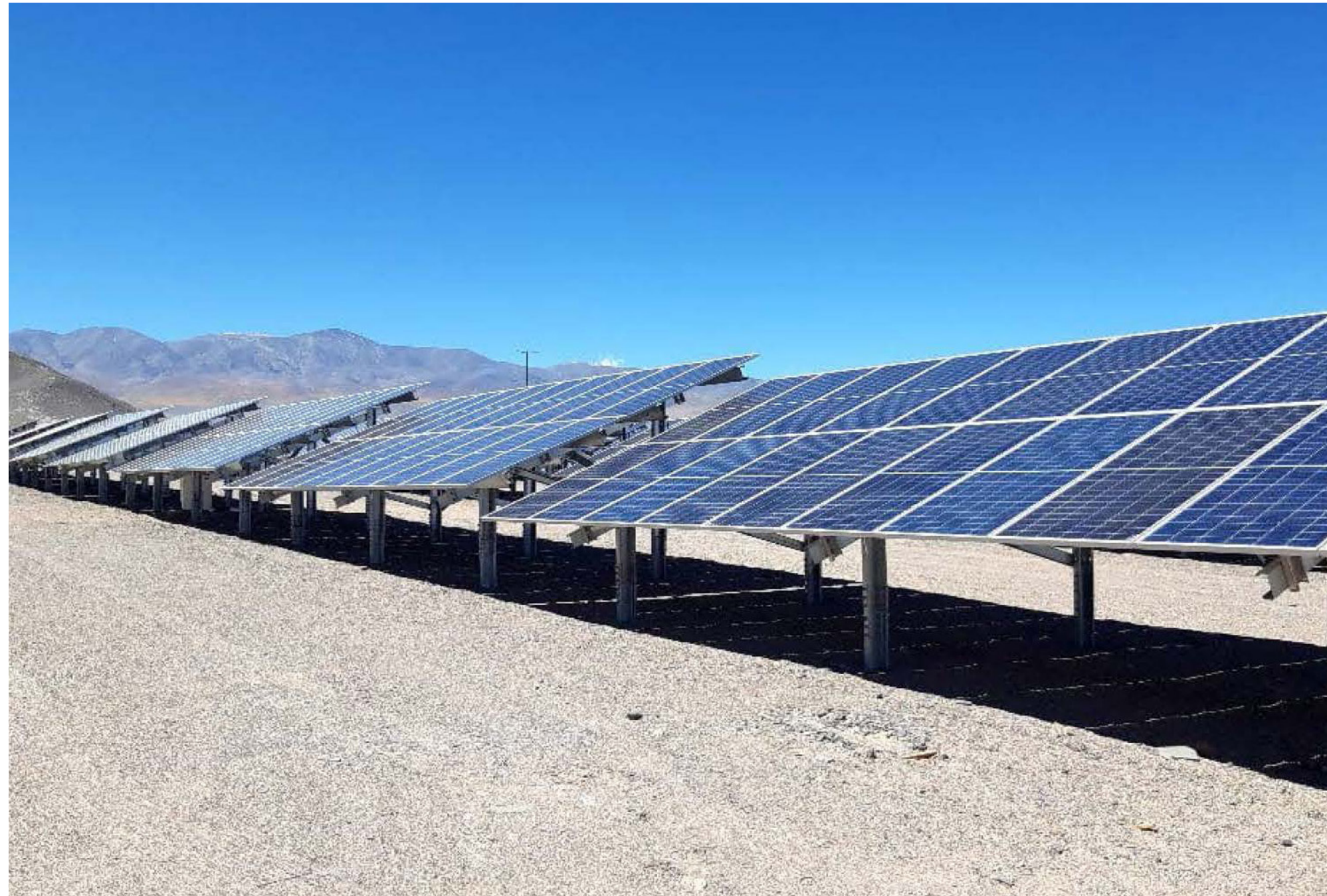
Solar park in El Peñon, Argentina, funded by the Water Trust
